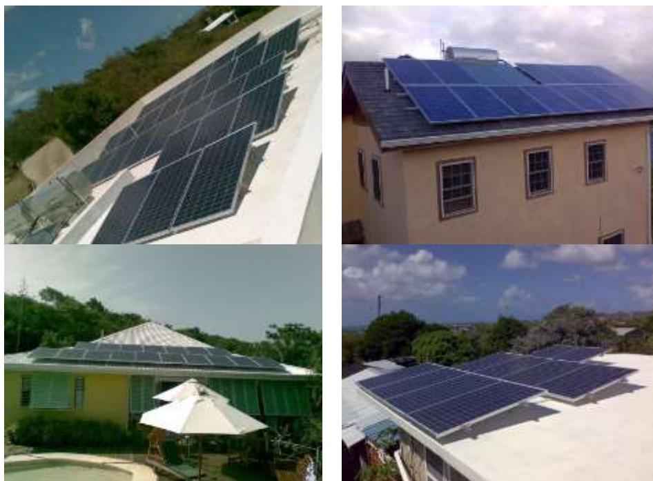
Figure 91-Photos of Installed Solar PV Systems in Grenada. Source: (GrenSol, n.d.)
