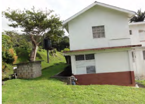
Figure 5.4: A section of the roof is concrete and adequate land space around building
