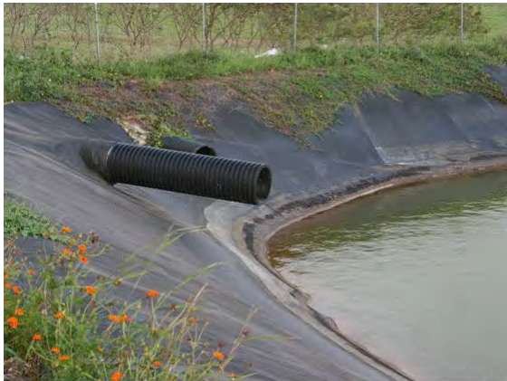
Tarpaulin RWH pond (Barbados)
