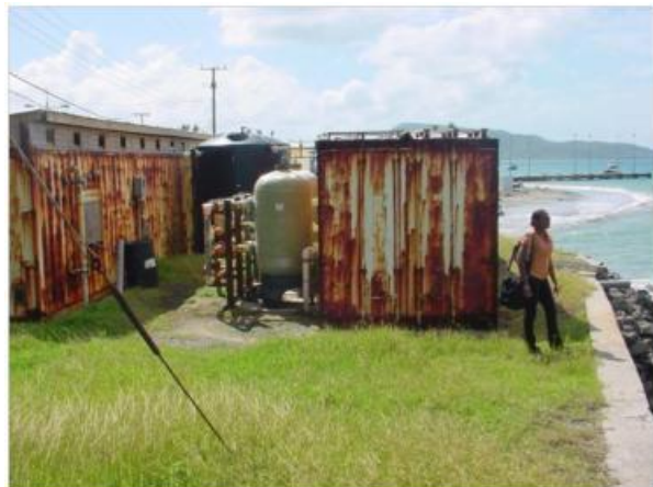
Figure 4.4: Derelict desalination plant at Petite Martinique subjected to harsh marine environment
