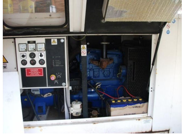
Figure 3.8: Backup diesel generator system at Carriacou's main hospital
