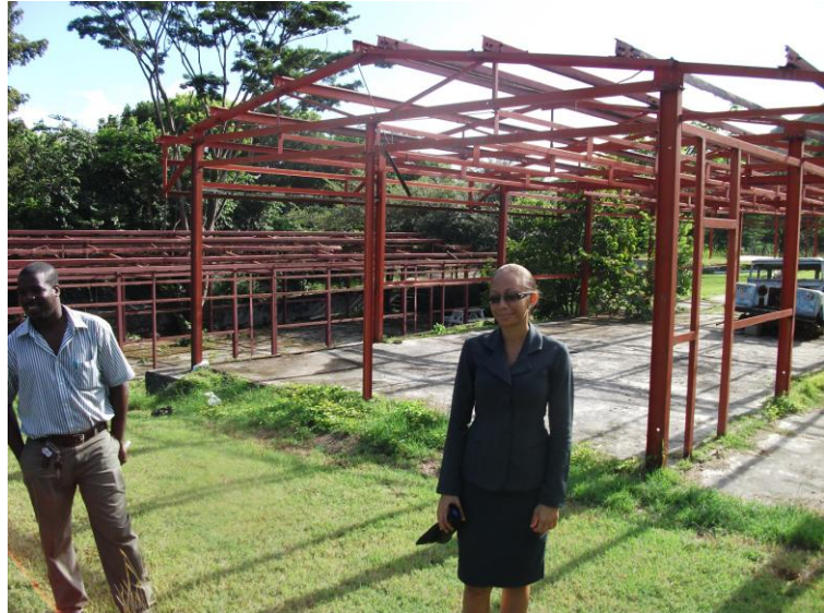
Figure 2.2: Unfinished facilities at T. A. Marryshow Community College
