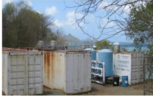
Figure 4.5: Abandoned desalination plant at Carriacou
