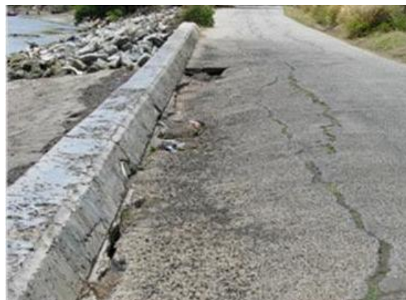
Figure 9.9: Protective sea wall and stone works threatened by coastal erosion at Windward, Carriacou
