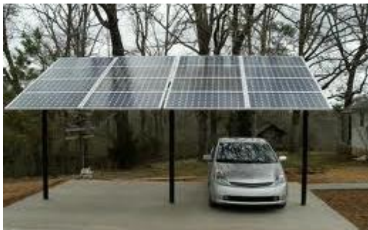
Figure 3.7: Solar PV carport (source: www.domesticfuel.com)
