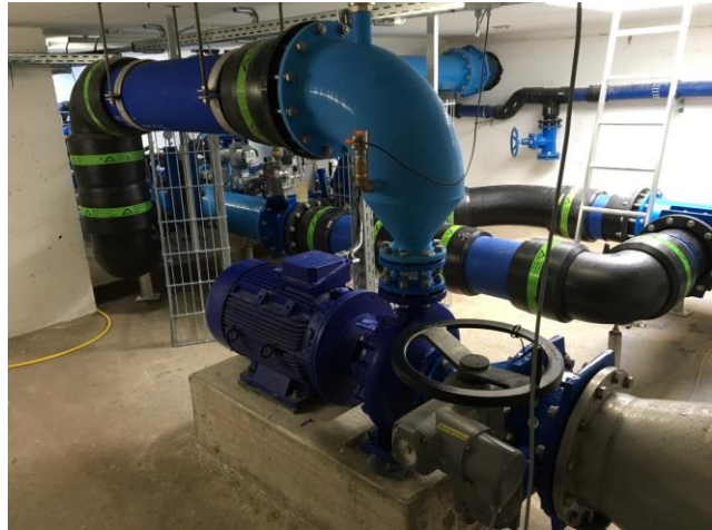
Pump as Turbine Wernigerode, Germany
